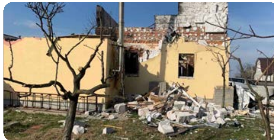
The war has caused significant and widespread damage to homes and infrastructure
